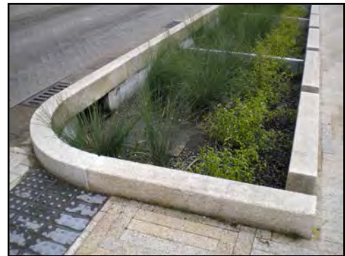
Fig. 3-27-BB: LID stormwater management feature
