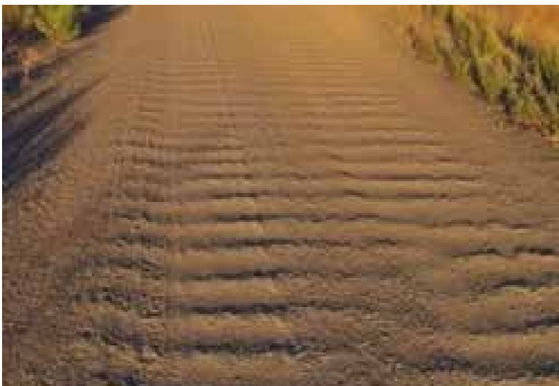
Figure 3.16: Washboarding (source: Landlock Paving)
