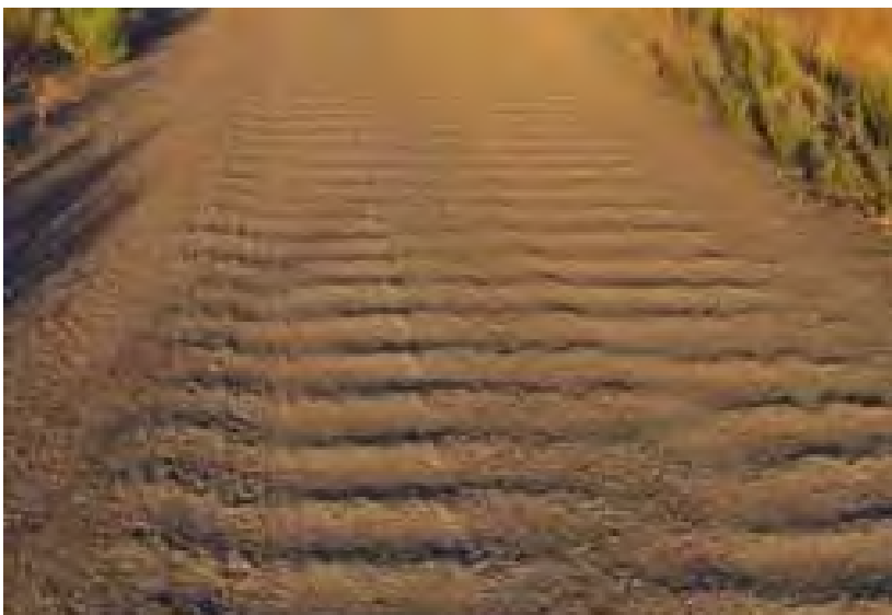
Figure 3.16: Washboarding (source: Landlock Paving)
