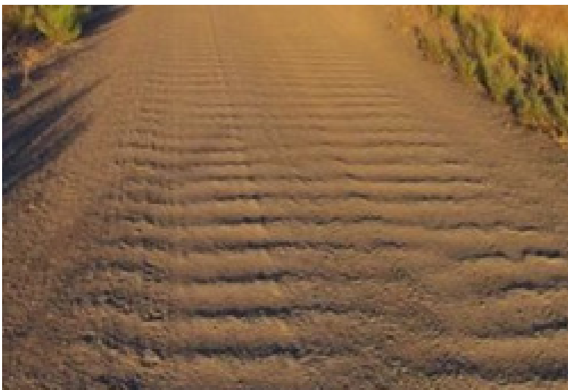
Figure 3.16: Washboarding (source: Landlock Paving)
