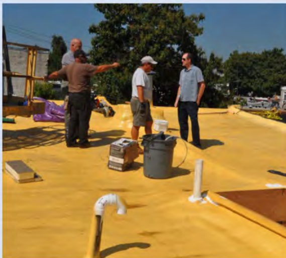
The Energy Coordinating Agency at work with EnergyFIT cool roofing repairs in Philadelphia, Pennsylvania.
