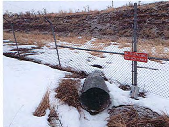
30" Storm Drain Outlet
