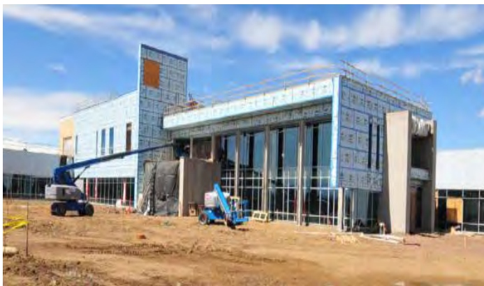
Construction on new Adams County Human Services Building in Westminster Colorado. On West side of I-25, on Huron Street near 120th Avenue.
