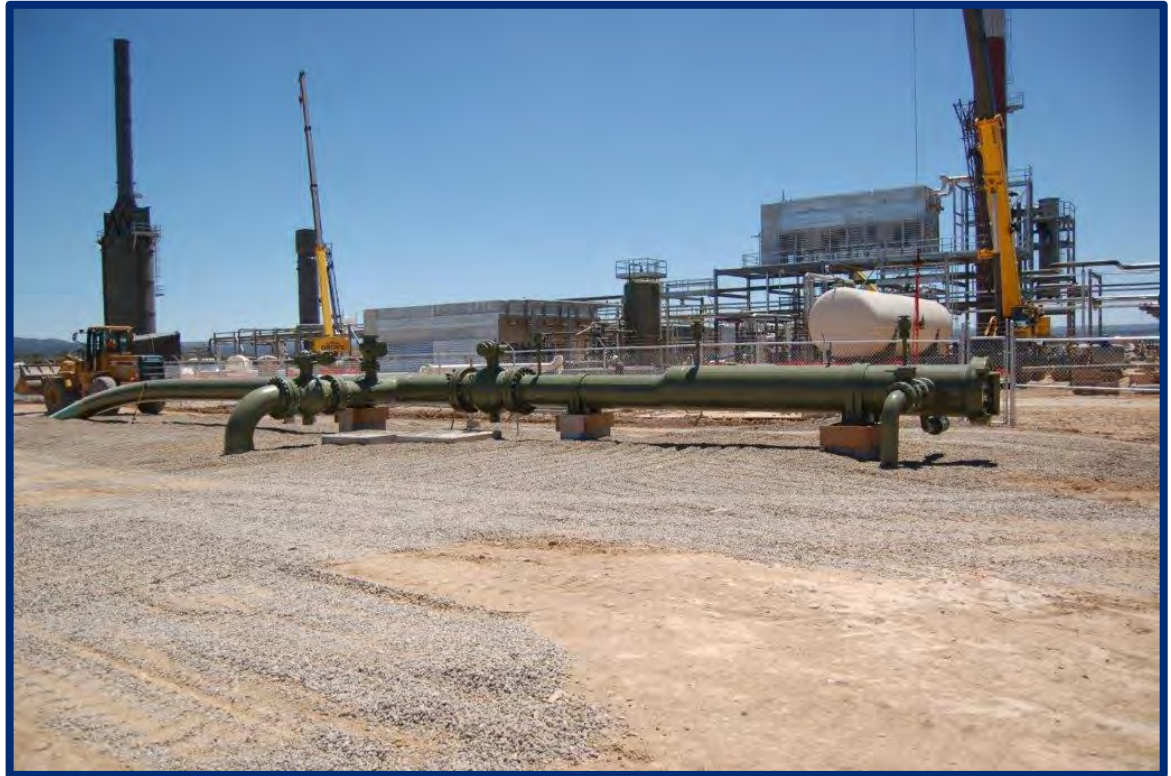
Figure 1.2.4 – Typical Pipeline Pig Receiver / Pig Launcher
