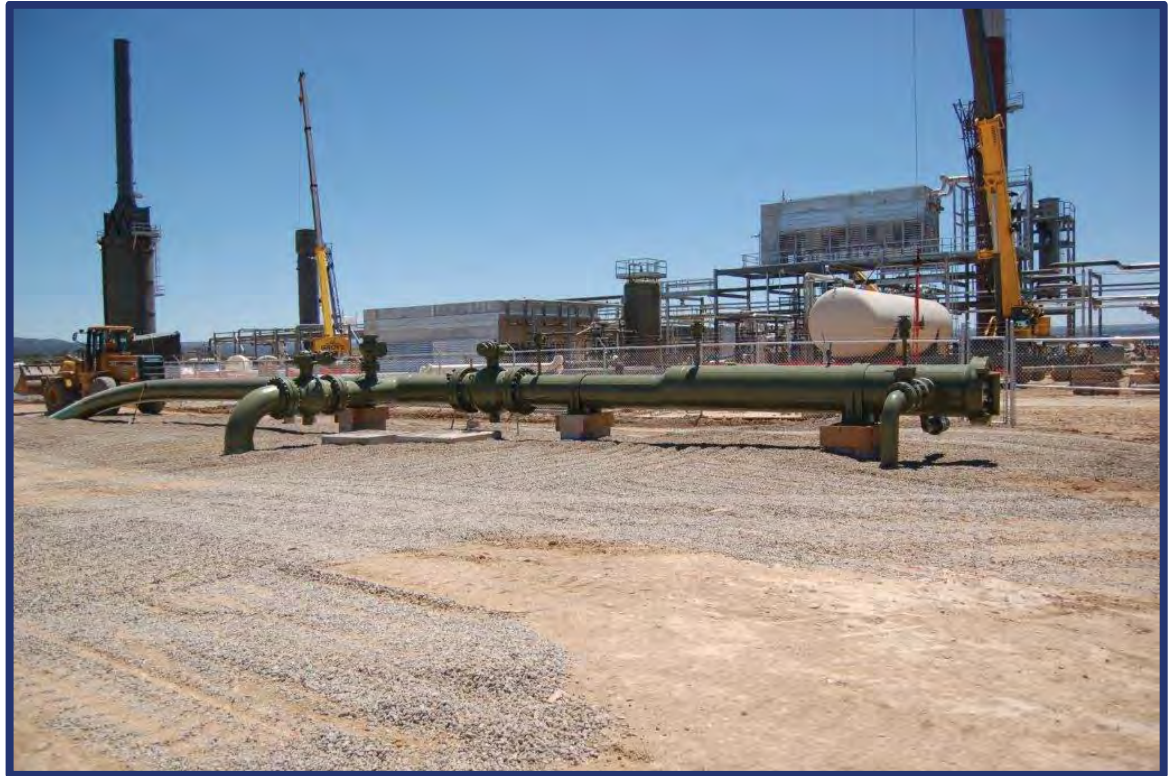
Figure 1.2.4 – Typical Pipeline Pig Receiver / Pig Launcher
