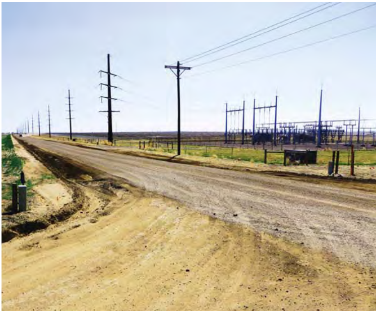
Existing IREA substation and transmission line.
