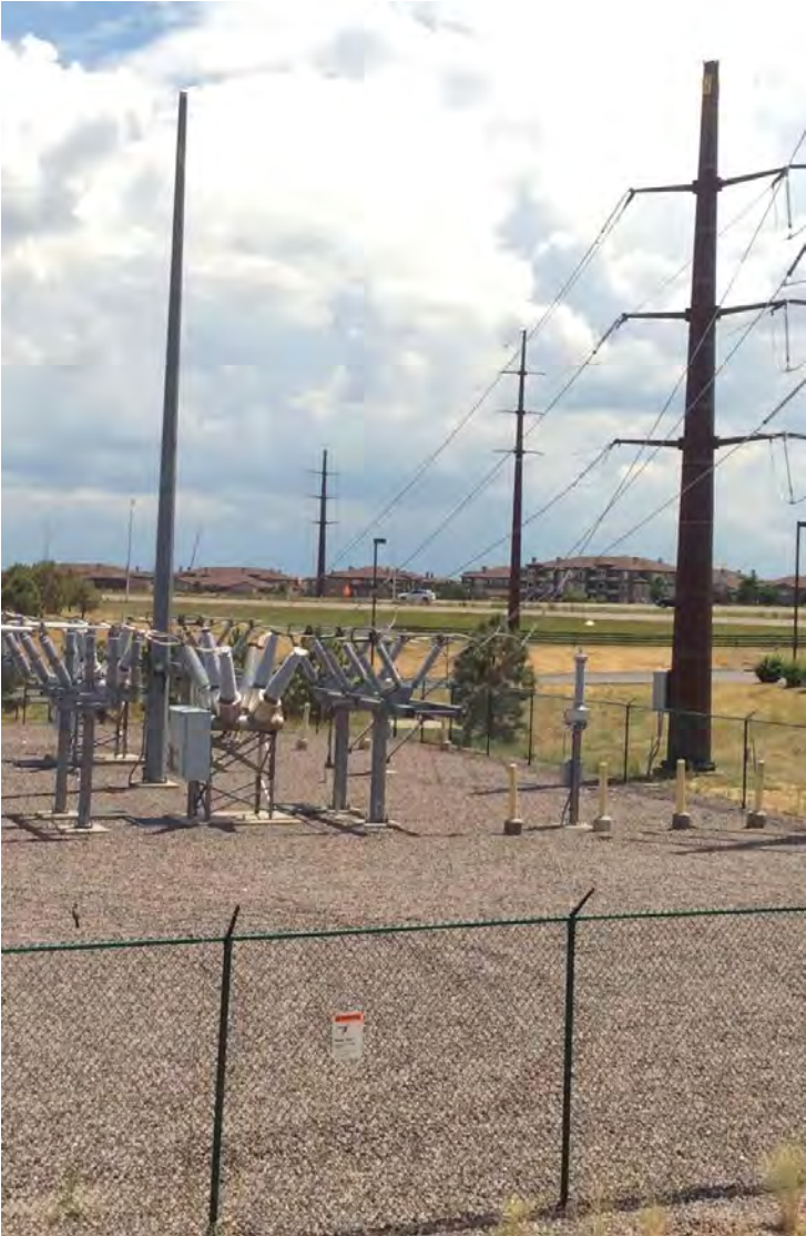
Typical Switchyard Breakers
