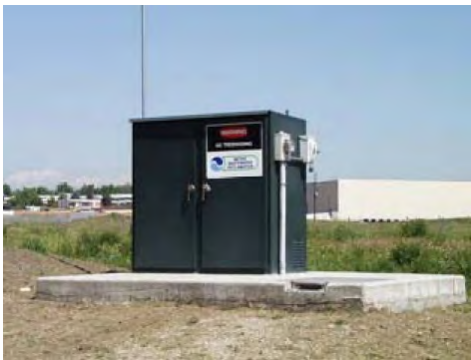
Example of Metering Station
