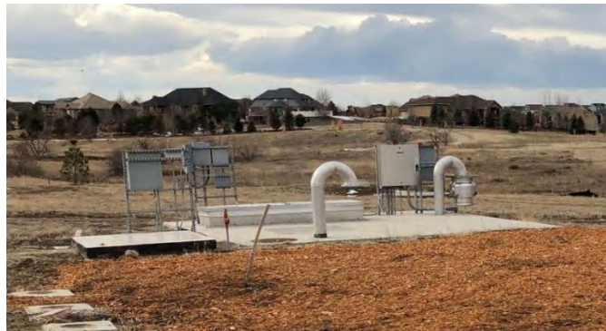
Example of Odor Control Facility
