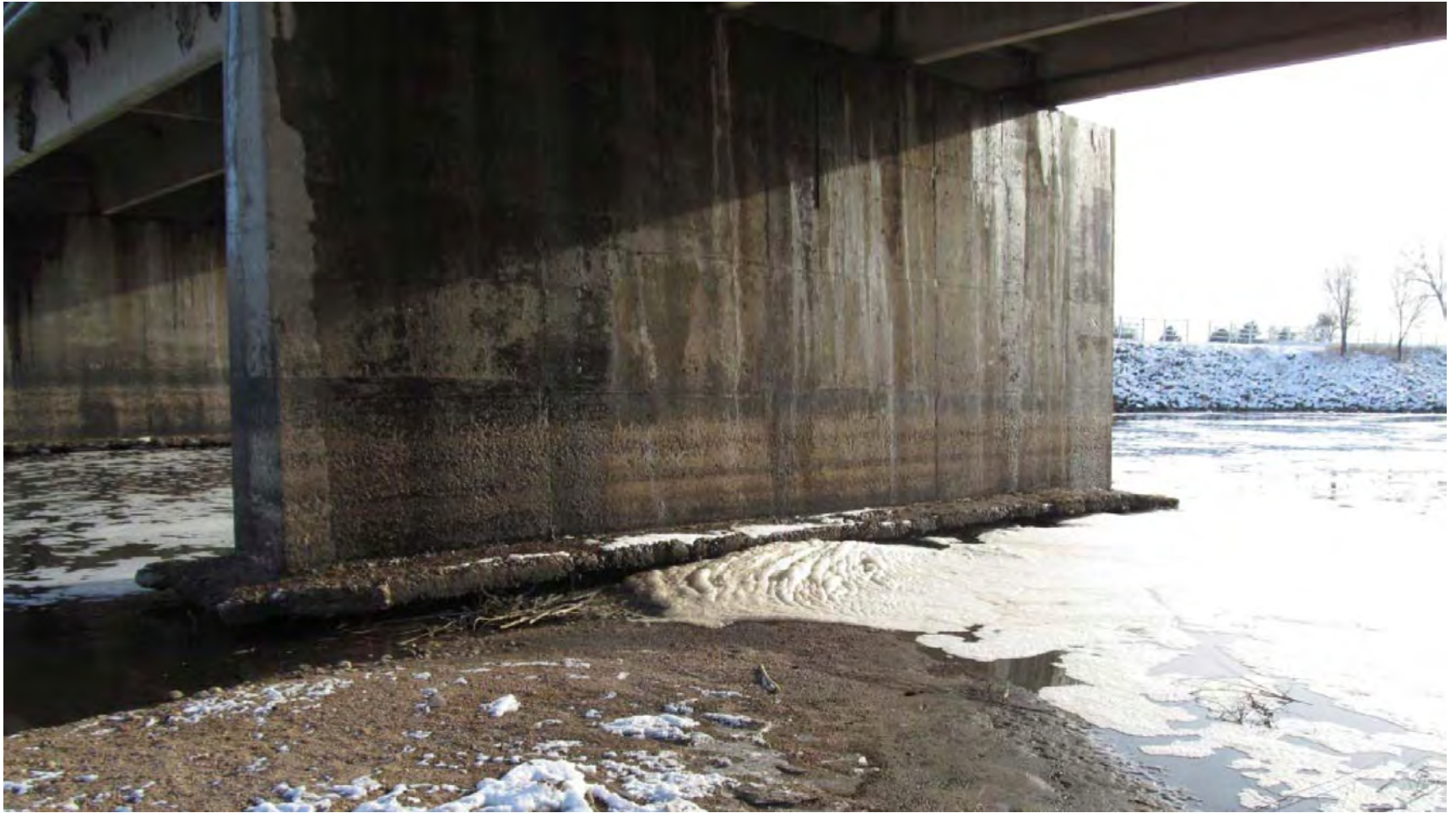
Pier 3 - Footing and Piles Exposed
