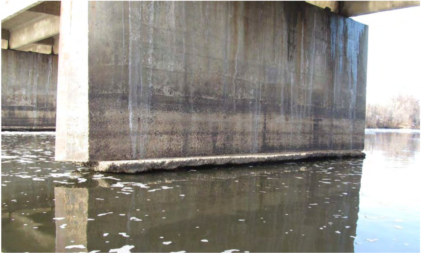
Pier 4 - Footing and Piles Exposed
