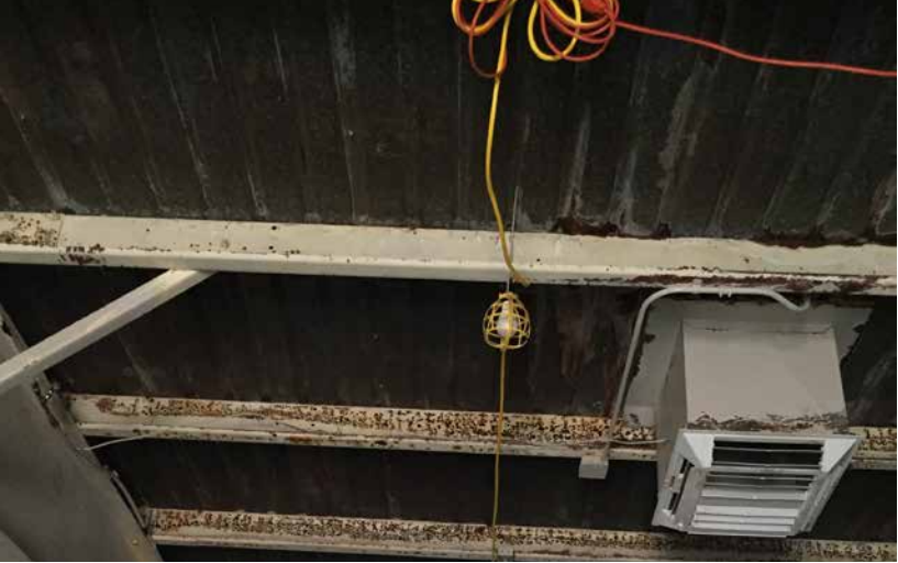
EXPOSED PLYWOOD PANELS TO KEEP OUT WINTER CONDITIONS, REMOVED IN SUMMER FOR VENTILATION
