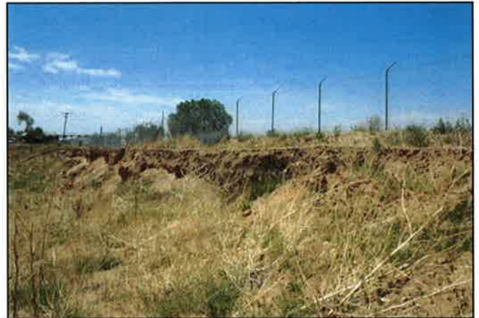
Figure 4 looking NNW @ the failure surface
