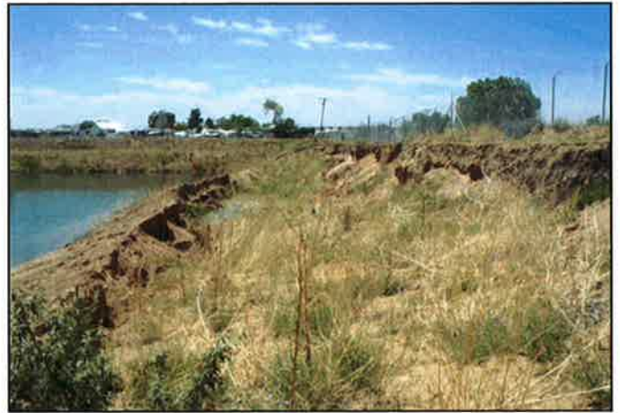
Figure 2 showing the area of embankment failure 5/15/12
