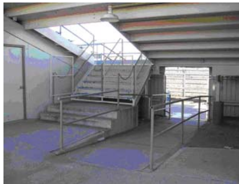
Main stair to Grandstand and adjacent portal for access to ADA seating and lower bleacher seating
