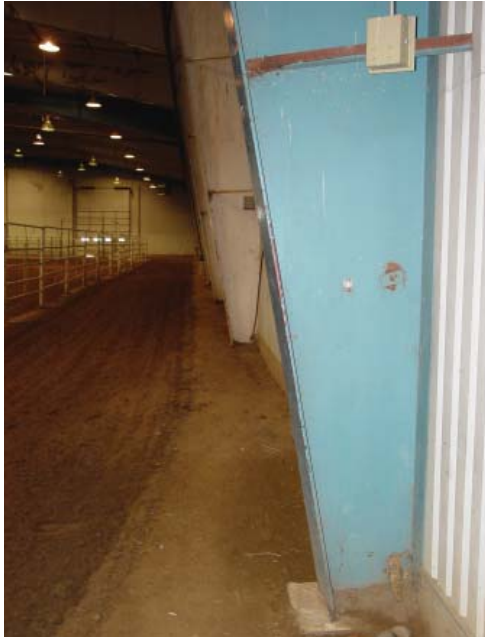
Structural frame showing corrosion
