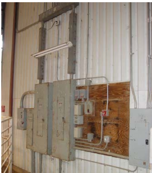
Main electrical panels
