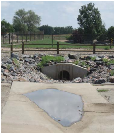
Grading issues at existing stormwater inlet
