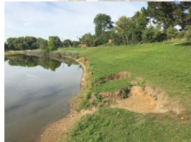
ERODED LAKE BANK
